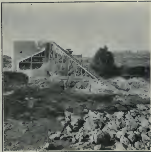
View of Lime Kilns and Hydrating Plant. Two more kilns under construction.
